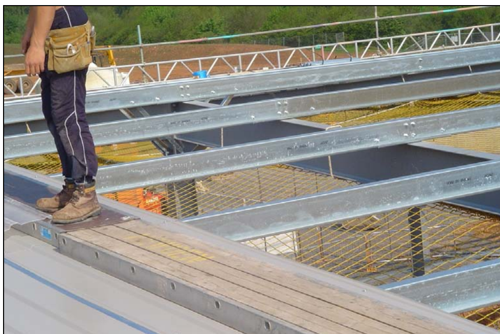
Figure 5.3 Safety nets and guardrail in place during roof cladding installation (Image courtesy of C A Roofing)
