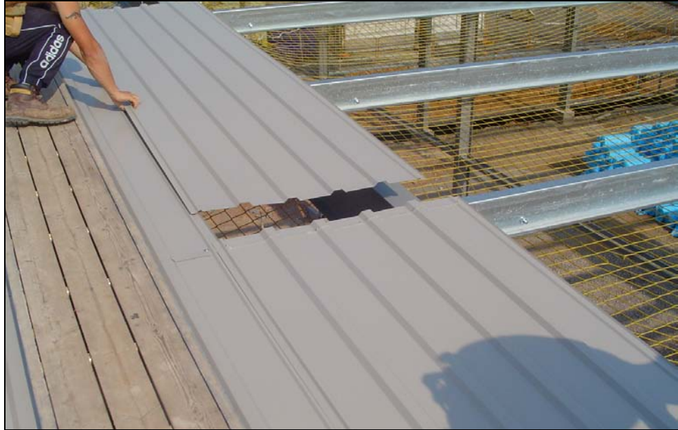
Figure 5.5 Liner sheet installation progressing into the span of the purlins with the installer working from a 'Youngman' board (Image courtesy of C A Roofing)
